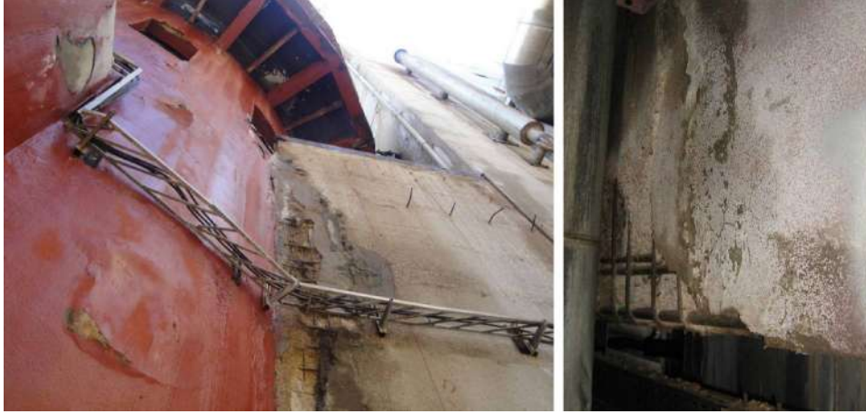
Fig. 3 Some examples of concrete destruction.
